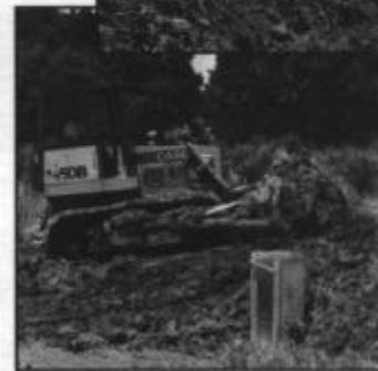
Depressional wetlands can be enhanced by shoveling levees closed (top), building up exterior levees with levee plows (middle) or installing water control structures (bottom).
